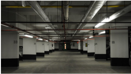
Replacing the metal halide fixtures in the underground parking with T8 LED fixtures provided a whiter light and cut 16,900 kWh.
